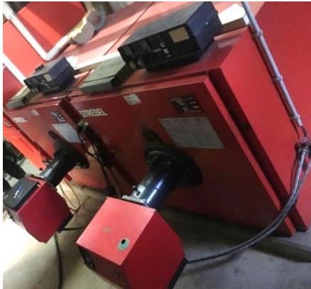
Figure 4 : Chaudières complexe scolaire
